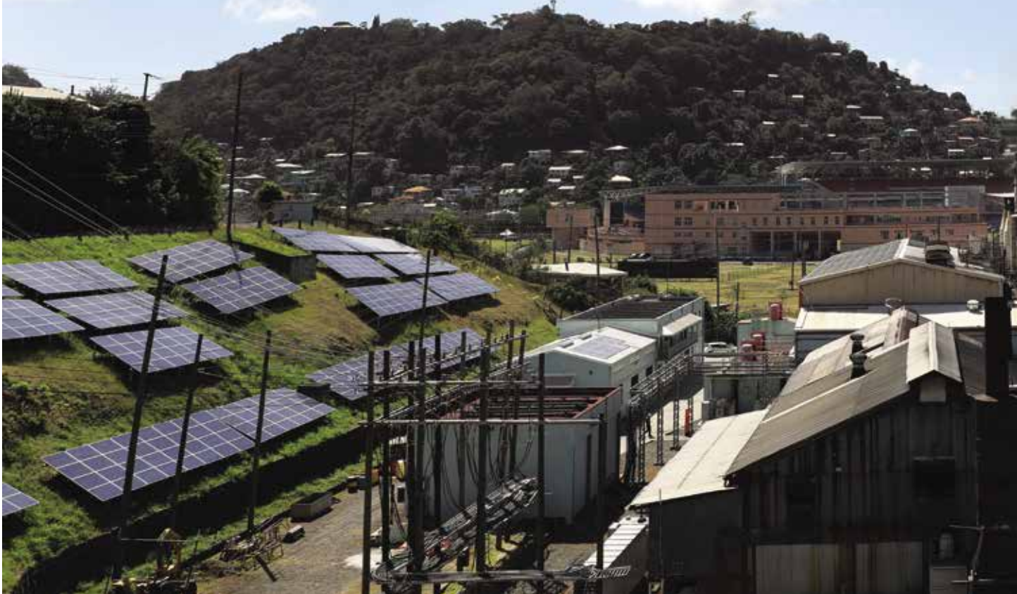
Using available land: hillside solar installation at Grenada Electricity Services (Grenlec), Grenada.
